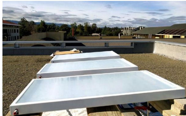
Figure 6. Rooftop sunlight reflection and air conditioning system
