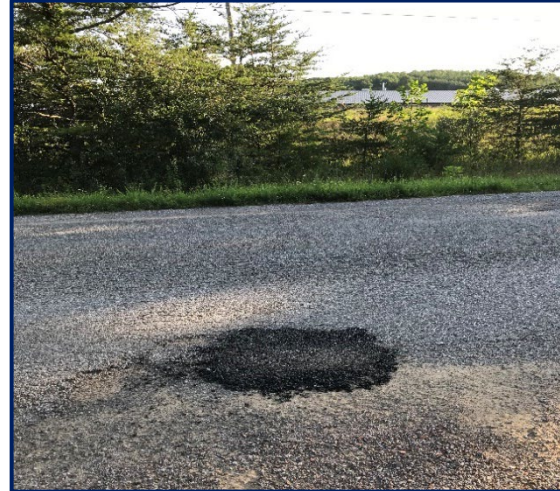
Filled potholes on non-county portion of Kelly Creek Road
