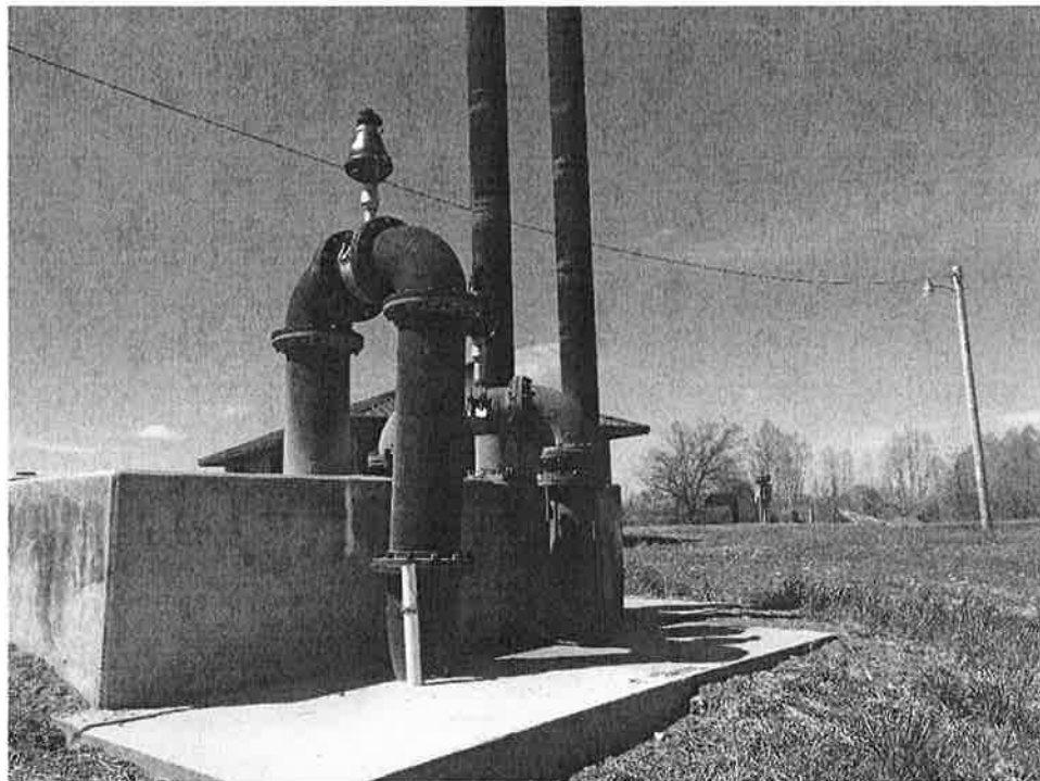
Figure 4 (2015). Three of the four incoming force mains entering the stilling chamber at the Tiptonville lagoon. Strap-on meters to be installed on vertical runs. Fourth force main not shown (installed in 2017 w/ augur screen).
