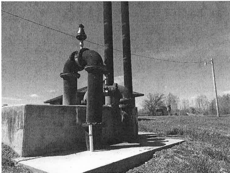
Figure 4 (2015). Three of the four incoming force mains entering the stilling chamber at the Tiptonville lagoon. Strap-on meters to be installed on vertical runs. Fourth force main not shown (installed in 2017 w/ augur screen).
