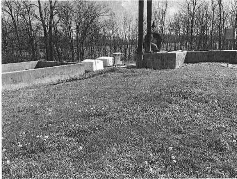
Figure 3 (2015). Photograph depicting three of the four incoming force mains entering the stilling chamber at the Tiptonville lagoon. Strap-on meters to be installed on vertical runs. Fourth force main not shown (installed in 2017 w/ augur screen).
