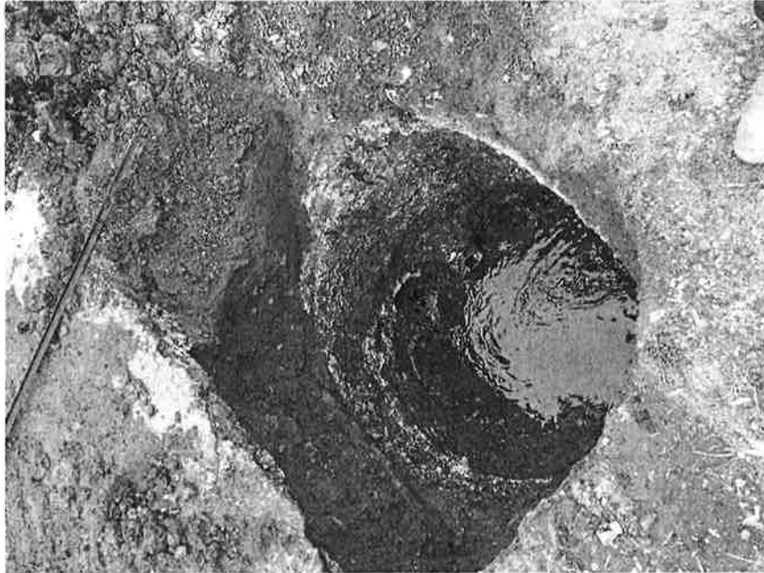
Figure 1. Photograph showing the condition of the Keystone St. manhole constructed in 1968.
